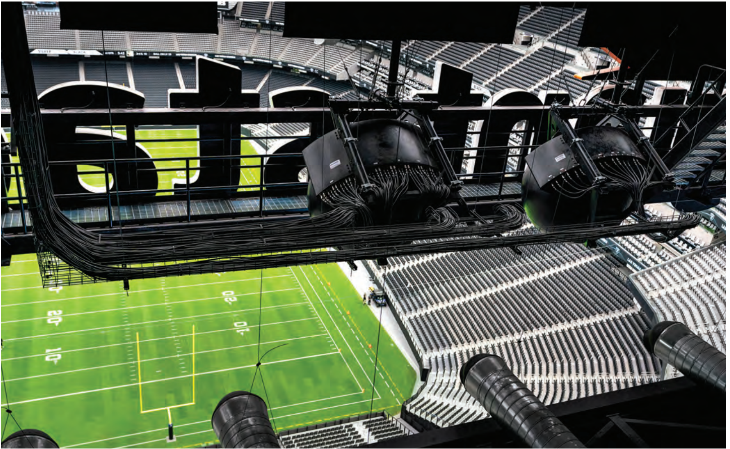
THE WELL-HIDDEN MATSING LENS ANTENNAS COVER THE SEATS BELOW WITH CELLULAR SIGNALS. CREDIT: MATT AGUIRRE/LAS VEGAS RAIDERS
