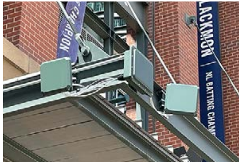
Extra Wi-Fi coverage was installed for exterior gathering places, like stadium entry gates
