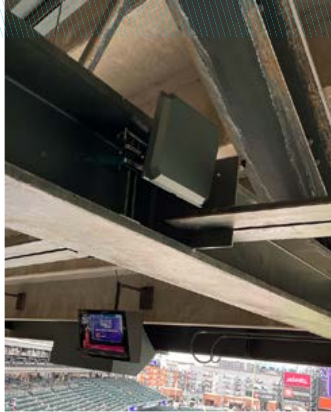
Wi-Fi antennas were moved out farther on overhangs to increase coverage.
